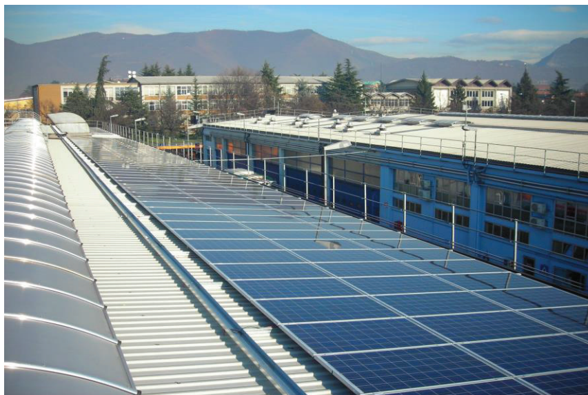
Fig. 5 Brescia Trasporti – The existing photovoltaic system installed in 2008
