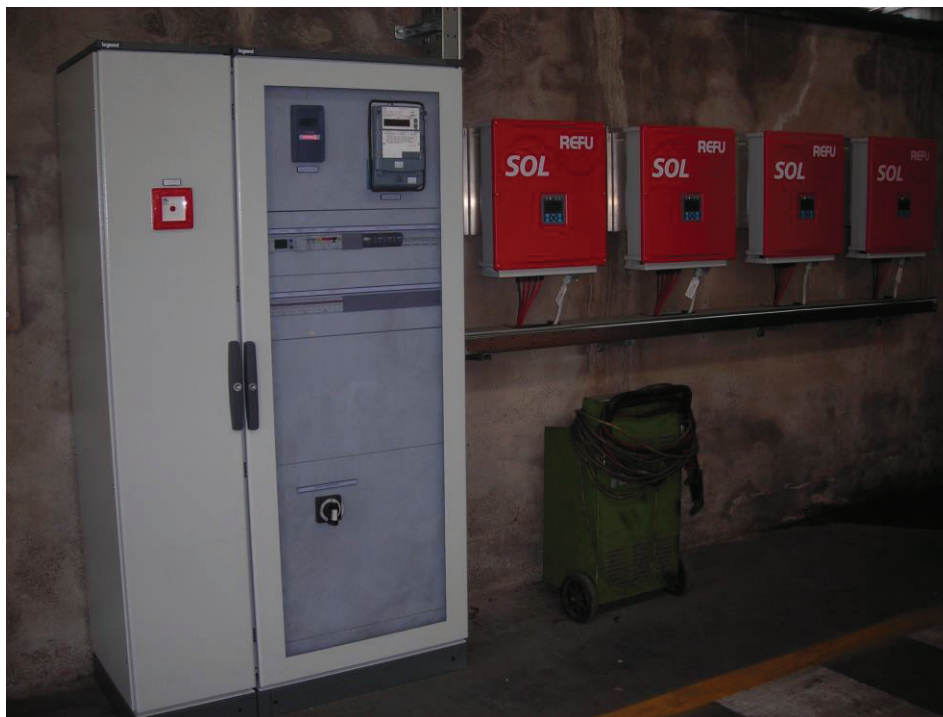
Fig. 7 Inverter and panel of the new photovoltaic system 76,8 kWp
