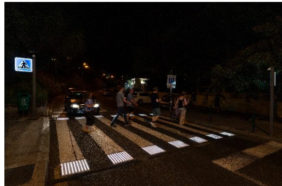
Figure 1: Integrated system implemented in Funchal that links road safety and energetic efficiency
