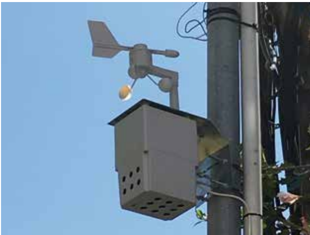
ReSEL environmental monitoring station for real-time air-quality monitoring
