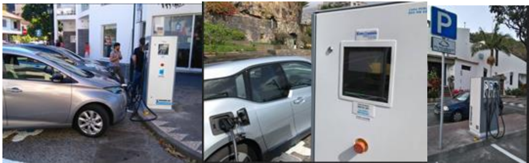
Figure 30: Fast e-charging stations installed in Madeira Public Network
