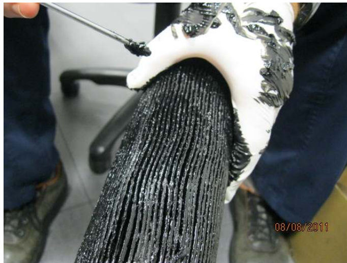
Figure 2: Dirty fuel filter
