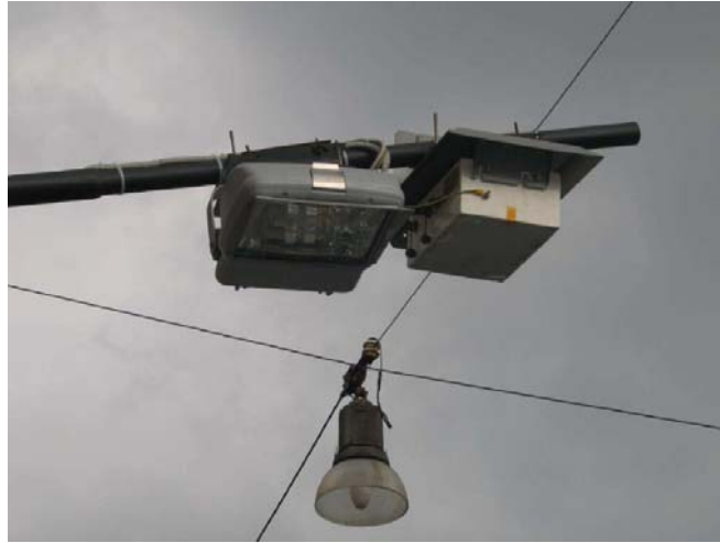
Figure 2: Fixed gate for bus lane control at Genoa
