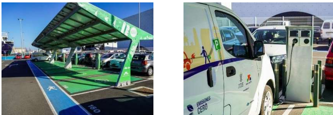
Figure 28 – EV charger stations at Muelle de Sanapú and Muelle de Sanapú parking facility.
