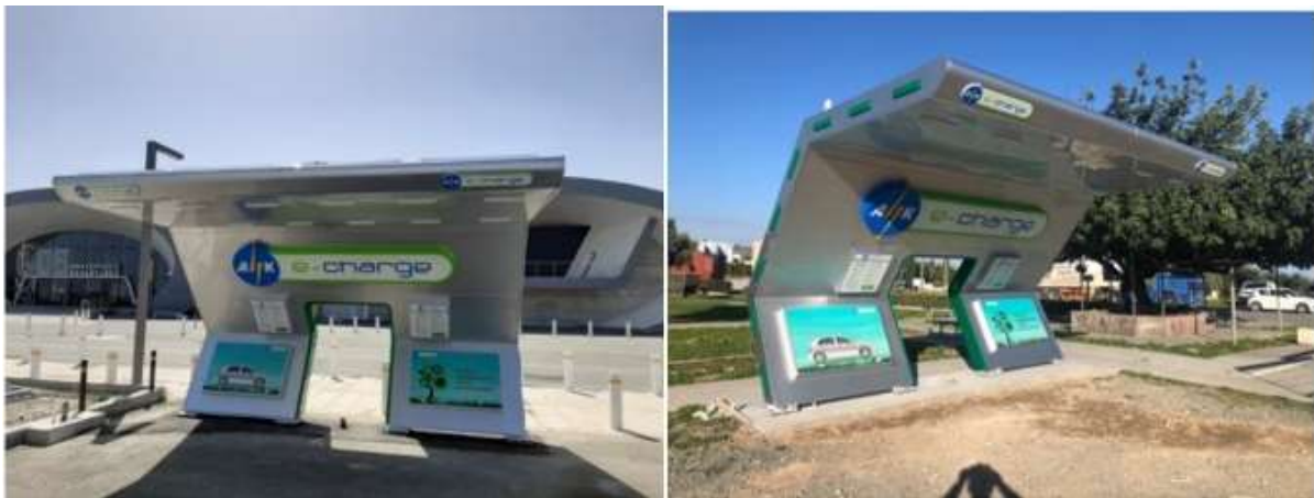
Figure 21 - Construction works for the installation of EV – Charging point with shelters at New Port and at the municipal Parking of Ypsonas Municipality
