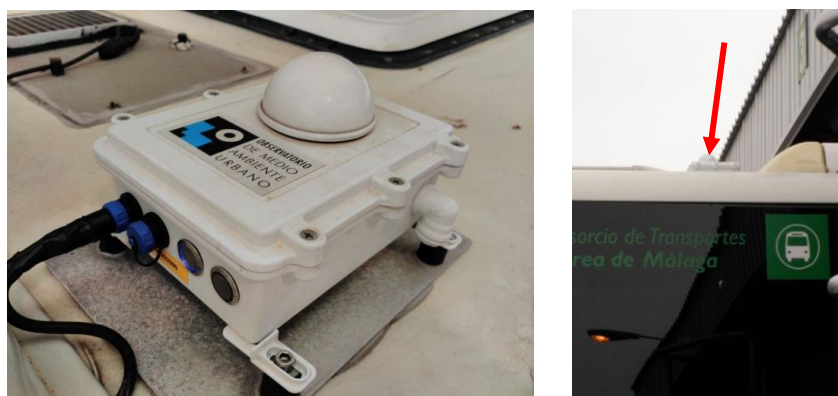
Figure 3: Example of a mobile station installed on a public bus
