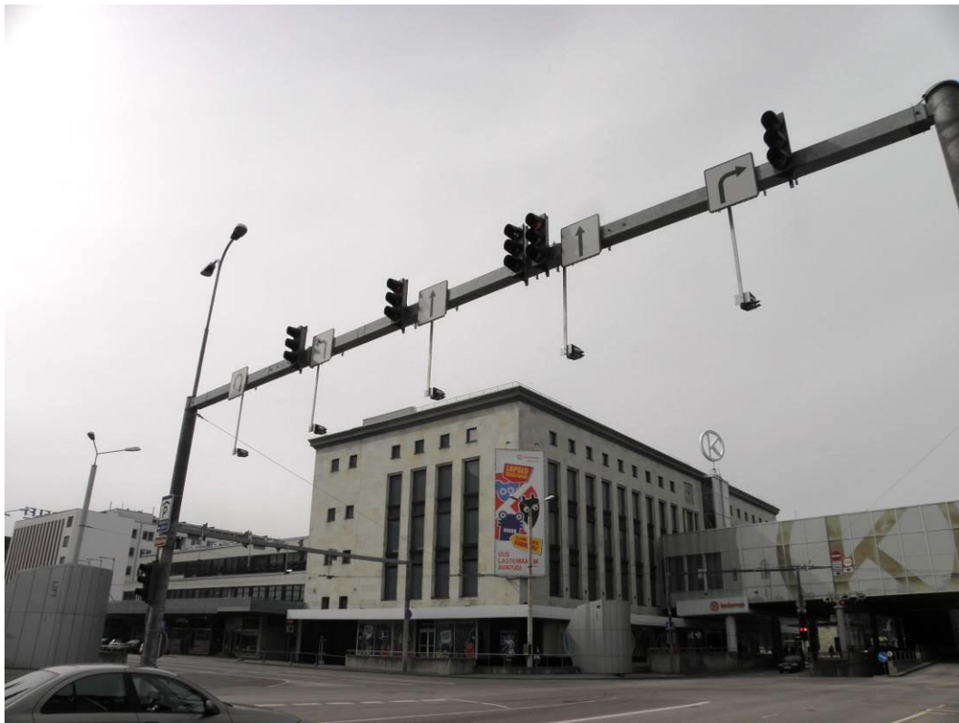
Figure 2 Monitoring cameras installed on the intersection no. 4
