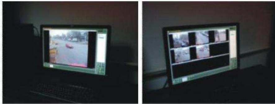
Figure 3 The dispatch centre – live real time video data from a single IP camera
