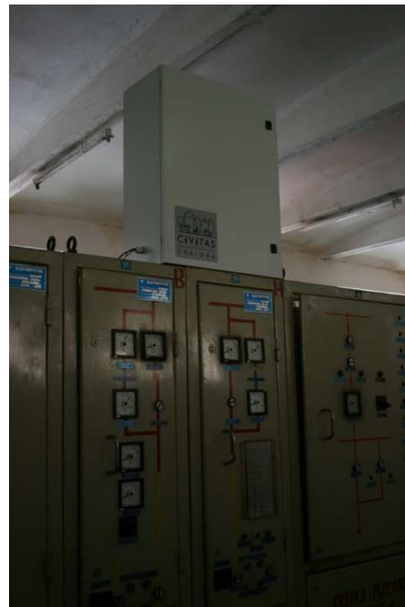
Data acquisition system from distribution stations
