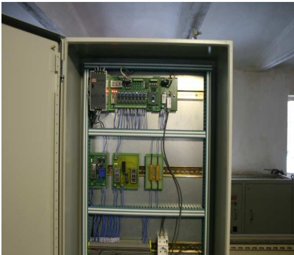
Metal cabinet with acquisition system
