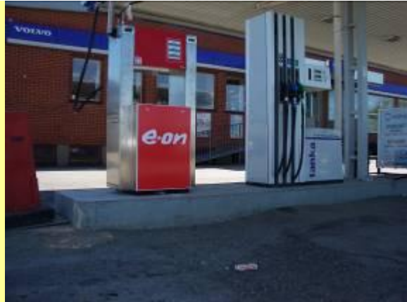
Picture 1C: The e.on CNG fuelling “pump” after connections were made with the CNG container storage.
