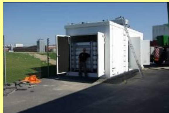
Picture 1B: View of interior of fuelling facility container storage of CNG.
