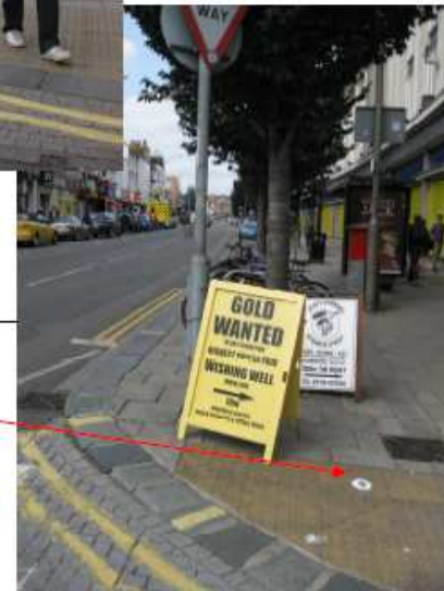
Illuminated no-entry sign positioning BEFORE
