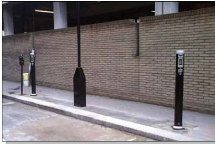
Integral feeder pillar and sign post installed with the Elektrobay
