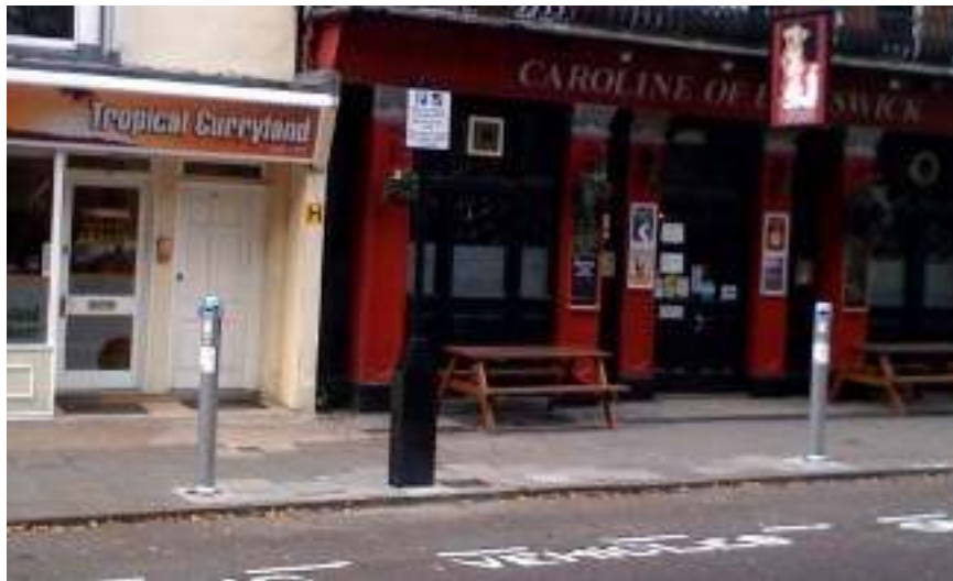
Figure 3: Charging Point in Ditchling Road, Brighton
