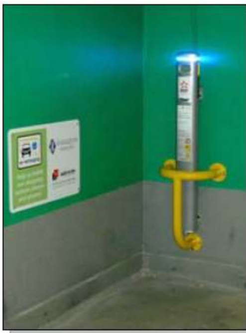
Wall mounted Elektrobay with barrier
