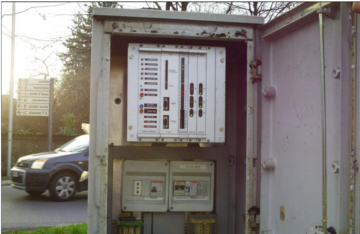
Figure 5 - Internal view of a Cabinet with a TLC in Monza
