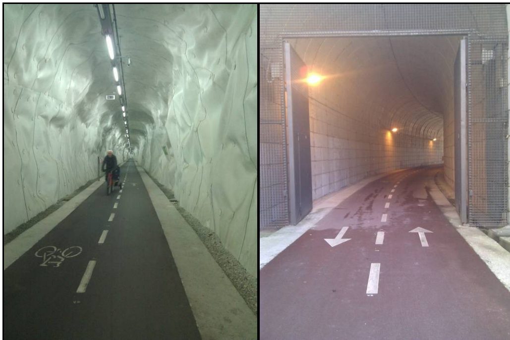
Figure 6: Large tunnel and short tunnel of Morlans, a part of the new cycling network.
