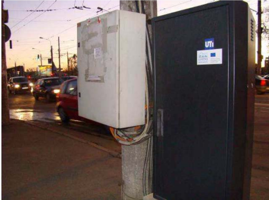
Fig. 4 Traffic light control system at a junction on the priority corridor
