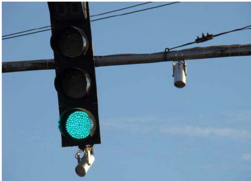
Fig. 3 Traffic signal and radar detector at a junction on the priority corridor
