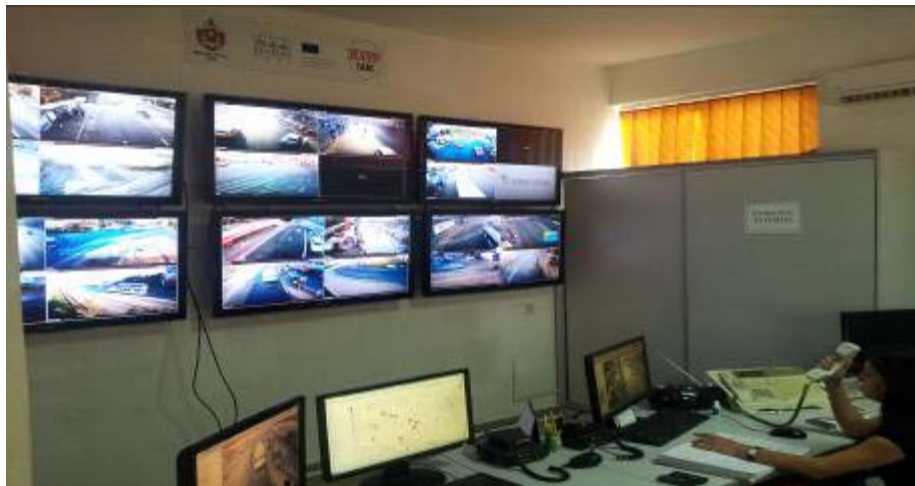
Fig. 3 The maintenance facility centre
