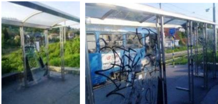
Damage and graffiti on bus station
