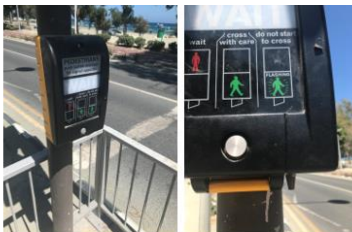
Figure 13: Traffic Signal System
