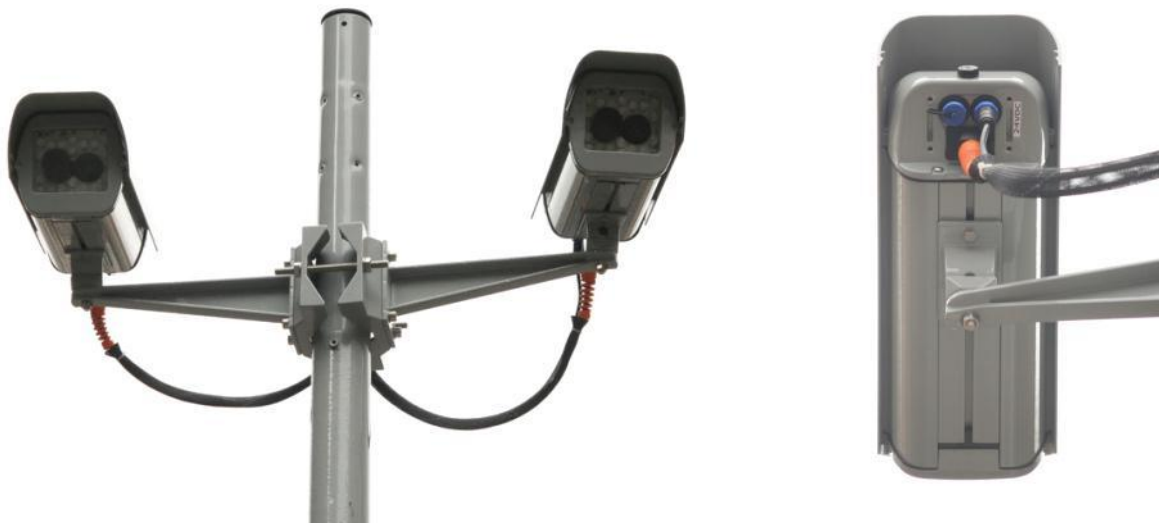
Photographs: Close-ups of the ANPR-cameras at St-Michielsplein
